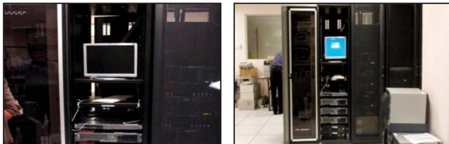
Gambar 10: ‘State Server’ TPC di Hospital Putrajaya
